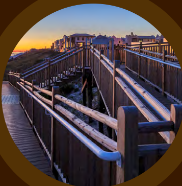
Wooden Pickets with ADA Grab Rails
