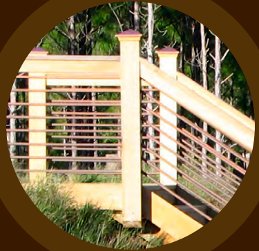
Horizontal Copper Tubing
